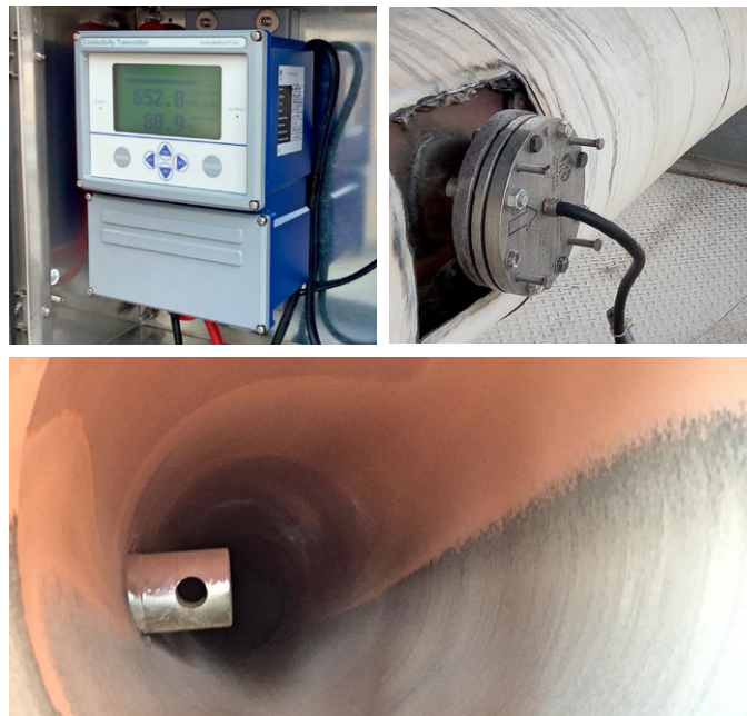
AL-DCIK FIELD INSTALLATION
