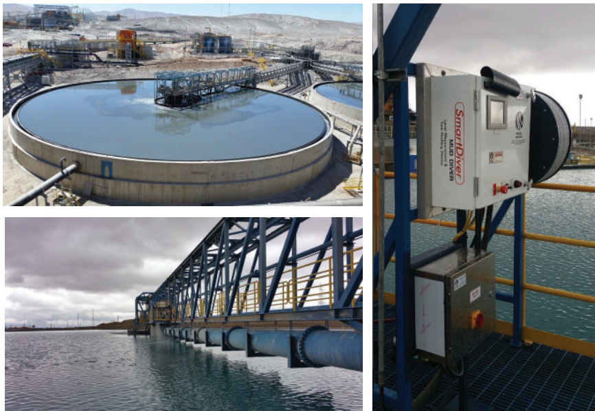
SMARTDIVER - COPPER THICKENER VESSELS APPLICATION
